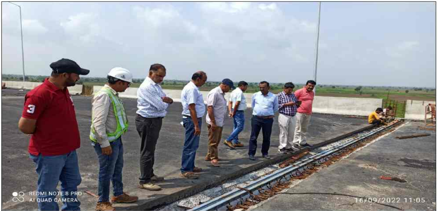
Team Leaders Site Visit at ROB, BC Laying Completed Expansion Joint Work in Progress
