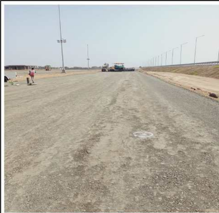
Ch.317+9 30 Truck Parking Area S.Road 317+900 to 318+070 Inner & Outer Edge DLC Laying Marking Complete RHS
