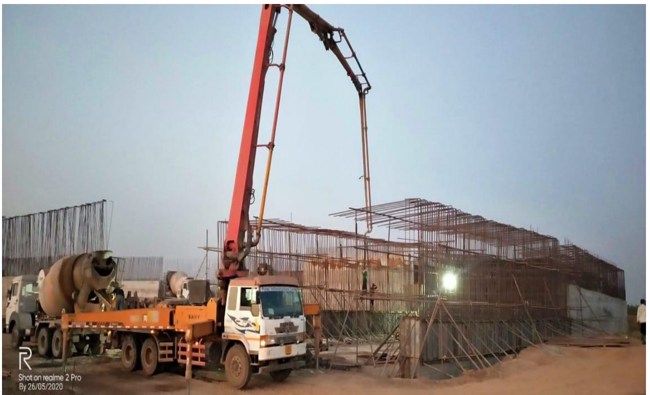
Ch-322+550 lhs pup A1 and A2 1st lift casting work in progress
