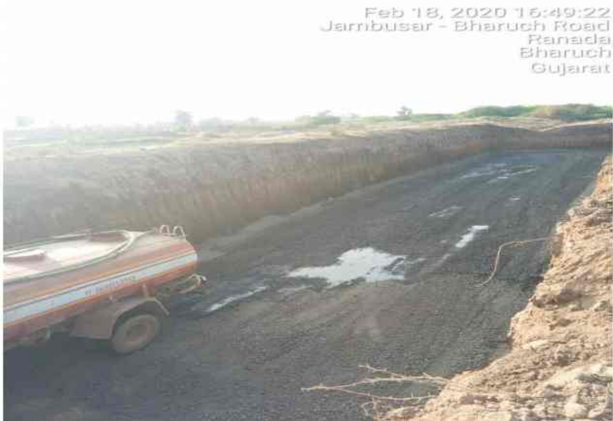
1st layer GSB bed water sprinkling work is going on at Chainage no 309+840 MNBA2 BHS
