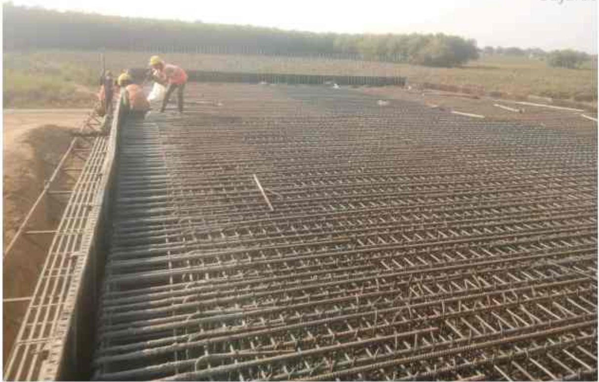
Shuttering fixing and lining & link bar binding work in progress at Chainage no 310+480 pup RHStop slab.
