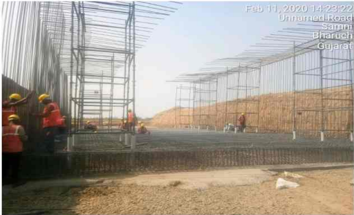
At Chainage no 306+820 pup RH Sraft top reinforcement binding with link bar work in progress. 1. Top reinforcement , 2. Extra bar binding, 3. Shuttering fixing remaining till now for raft concreting.
