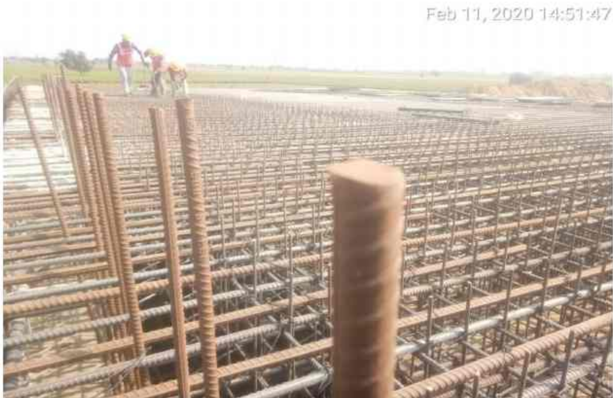
At Chainage no 308+550 LVUP RH Stop slab reinforcement binding and link binding work in progress. 1. Crash barrier reinforcement binding 2. Link bars & inner vertide bending 3. Both side shuttering fixing and lining 4. Haunch shuttering fixing and lining work is remaining till now.
