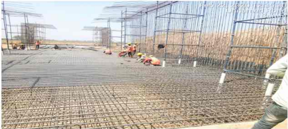
At Chainage no 306+820 pup LHStop reinforcement binding for raft work in progress.
