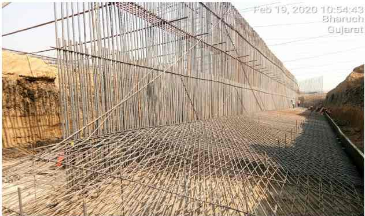
AT CHAINAGE NO 310+725 MNB A1 RHS REINFORCEMENT BINDING AND SHUTTERING FIXING WORK IN PROGRESS FOR RAFT.
