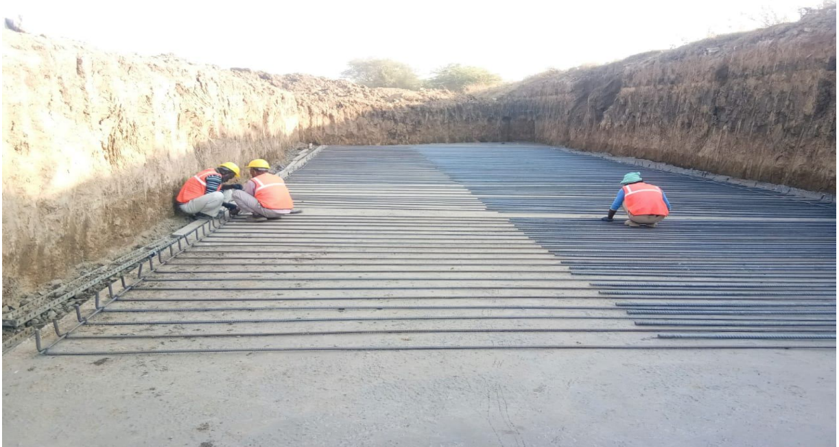
DT.29.01.2020 At Chainage no 313+840 MNB RHS A2 bottom reinforcement binding for raft work in progress .
