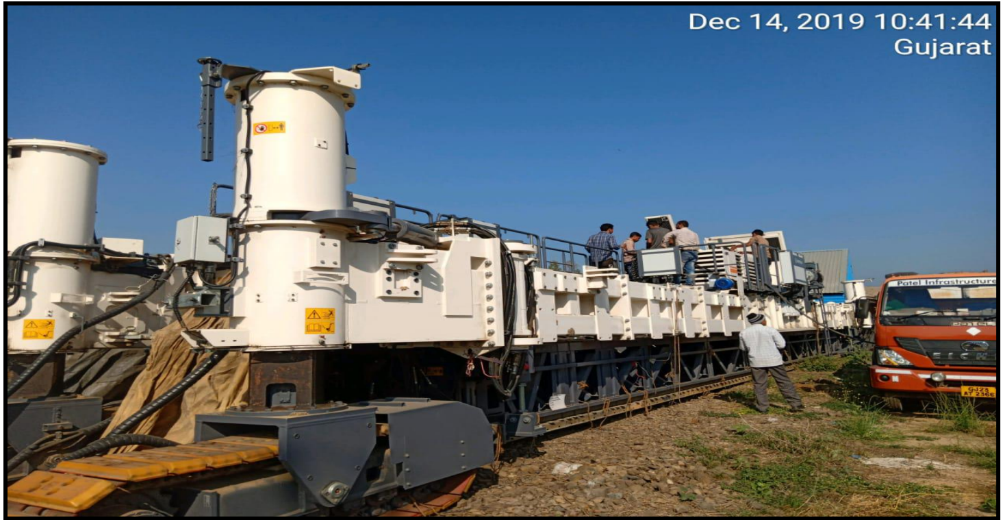
PQC PAVER ENGINE STARTING AND CHECKING THE WORK IN PRESENCE OF WIRTGEN SERVICE ENGINEER....
