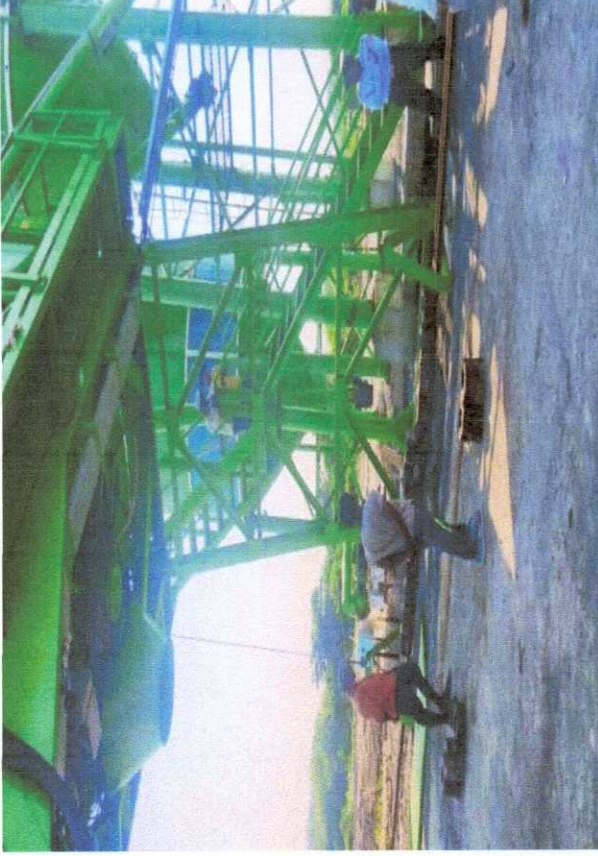
CALIBRATION OF M1C PLANT PIL CAMP
