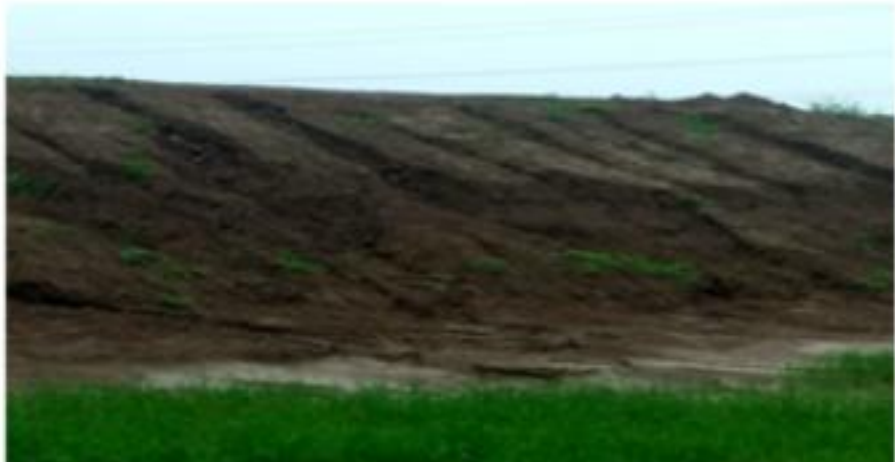
RAIN CUTS BETWEEN 324+250 TO 324+380 DATE 08.08.2019
