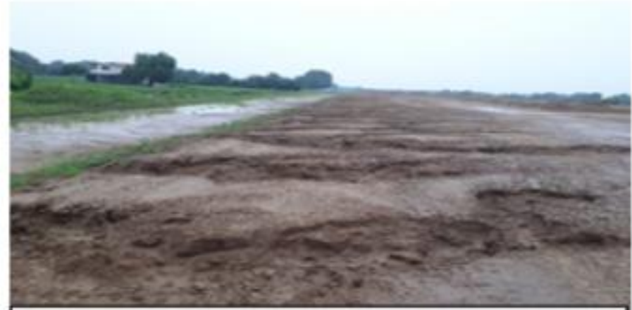
323+220 RAIN CUTS DATED 09082019
