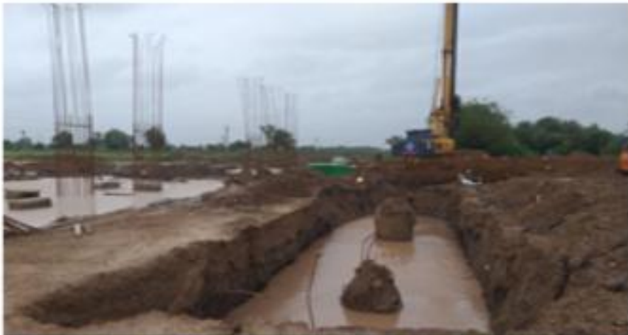
353+666 INTERCHANGE FLOODED DUE TO HEAVY RAIN 10.08.2019
