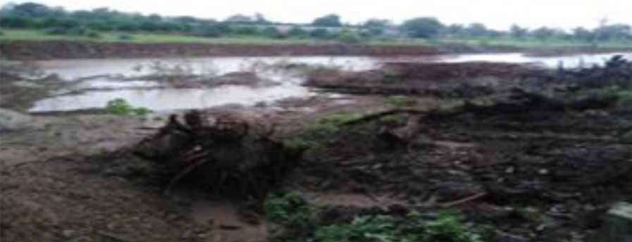
344+383 FLYOVER WROKING SITE FLOODED 10.08.2019
