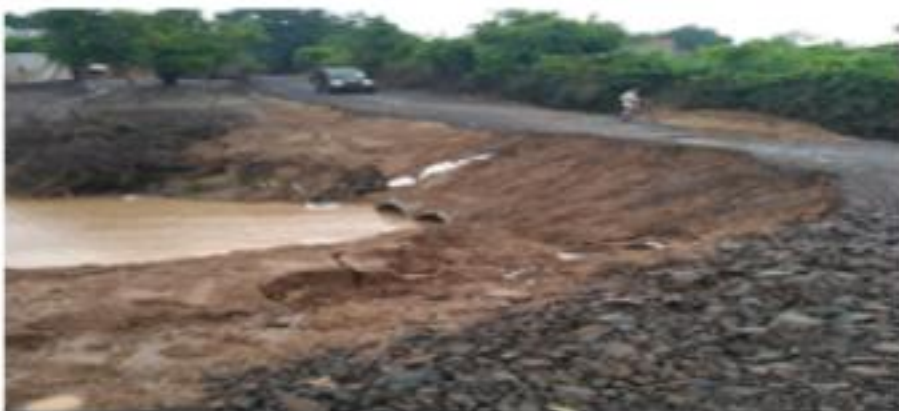
APPROACH ROAD FOR MAJOR BRIDGE DAMAGED DATE 09.08.2019
