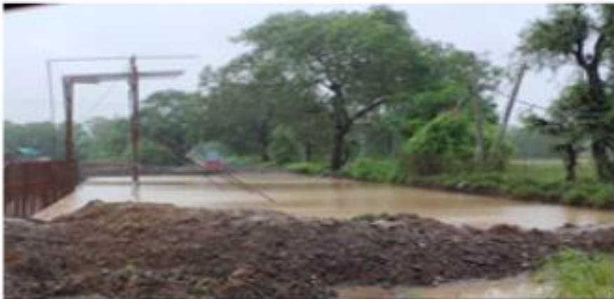
343+856 LVUP FLOODED WITH WATER DUE TO RAIN 11.08.2019
