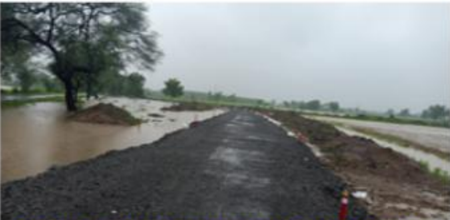
326+957 VOP DIVERSION DAMAGED 09082019
