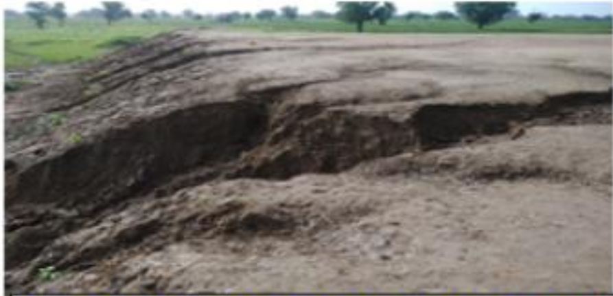
Ch. 329+500 to 329+800 EMB. BED WASHED OUT
