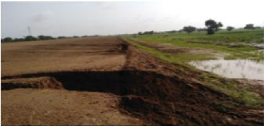
329+400 to 329+500 BHS BED ERODED BY RAIN CUT
