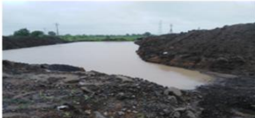
339+687 CUP FLOODED DUE TO HEAVY RAIN FALL 10.08.2019
