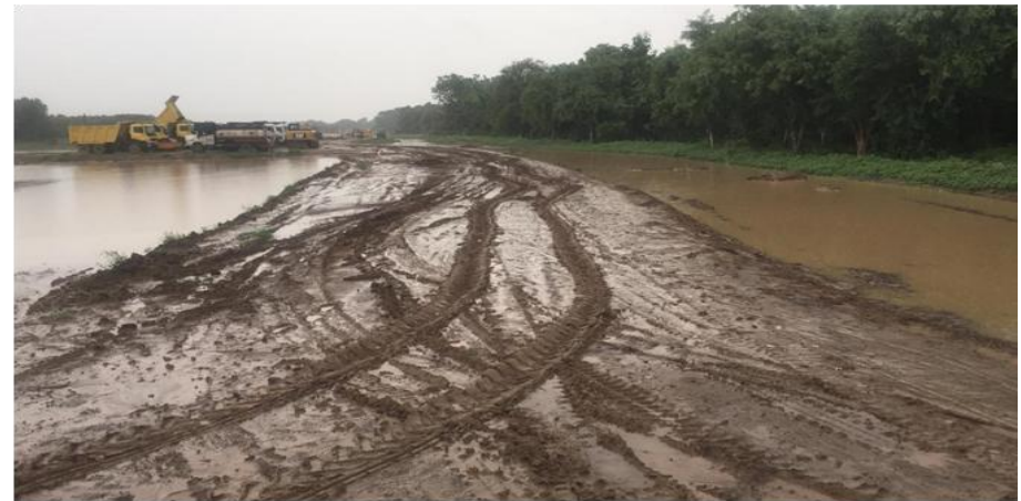
Ch. 349+220 - water logging due to heavy rain
