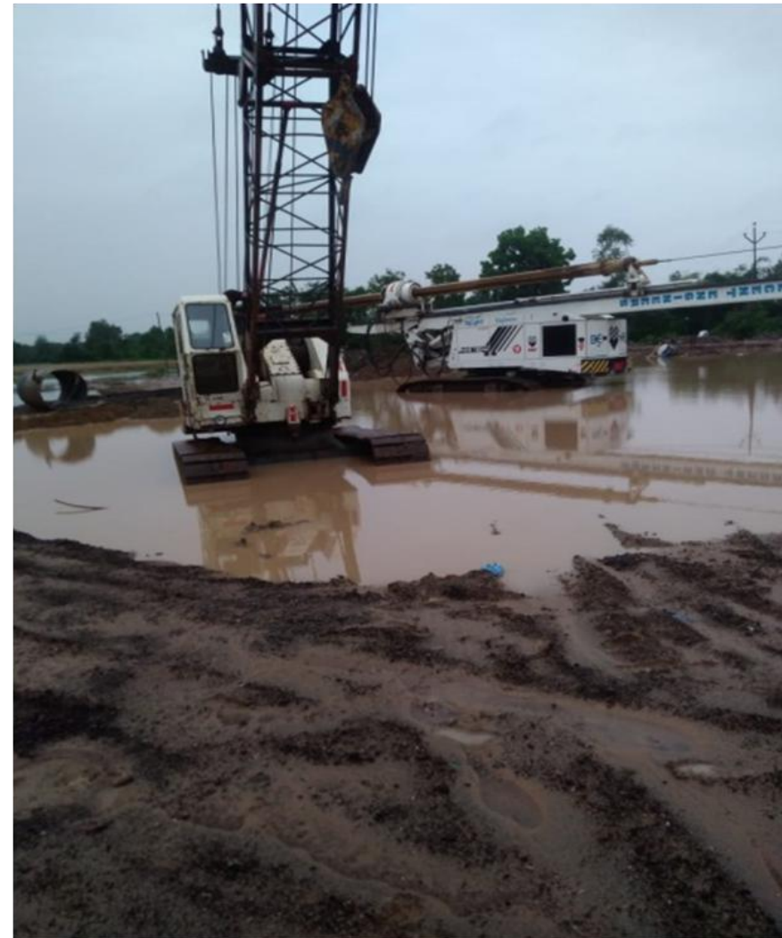
Ch. 353+666 - Heavy rainfall at Interchange
