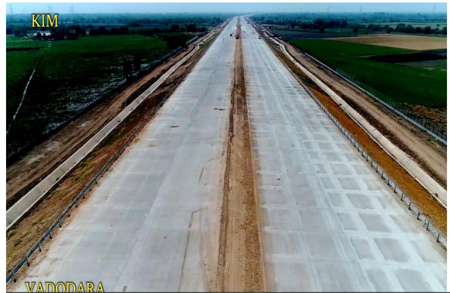
Road Status PQC, Pre cast U Drain, Toe Drain, MBCB at Km 338 to 339
