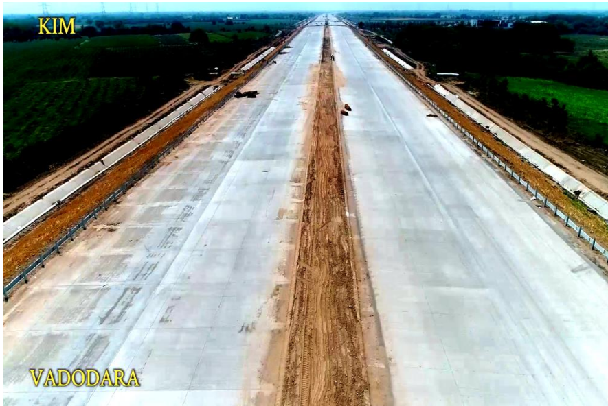
Road Status PQC, Precast U drain, MBCB, Slope Protection, Toe drain at 339+800
