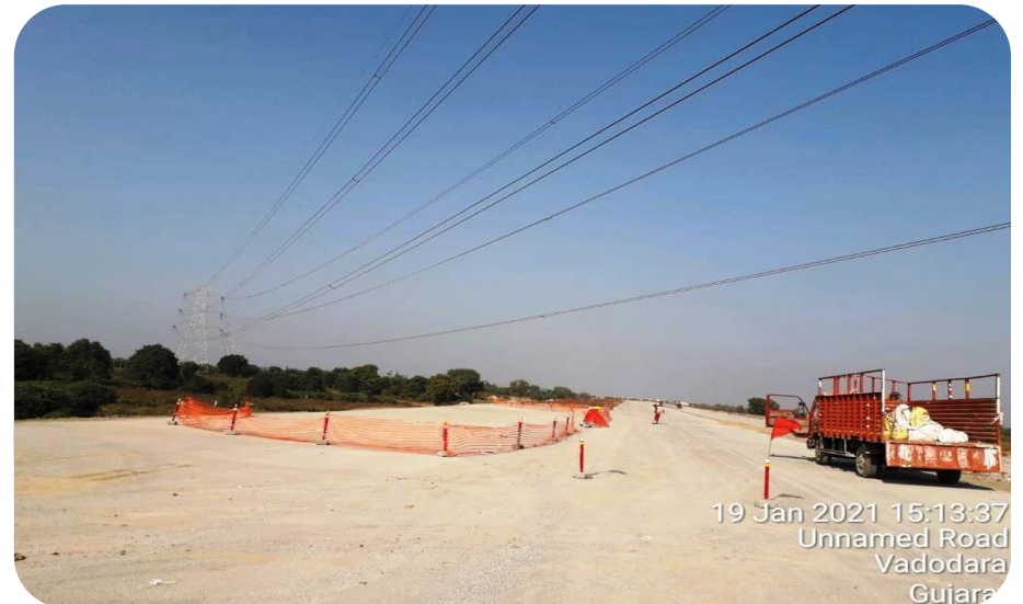
Overhead power line net barricading & red flag for indication at MJB ch-336+100
