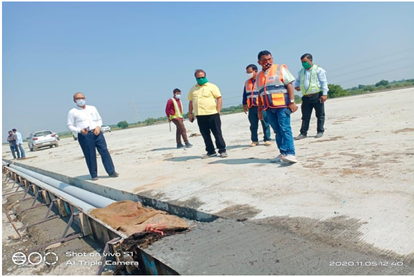
Quality inspection of Expressway by Concessionaire, work of utility duct in progress
