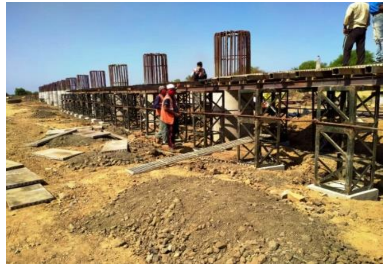
343+566 MNB PIER CAP SIDE STAGING AND BOTTOM PLATE PLACING WORK IS IN PROGRESS
