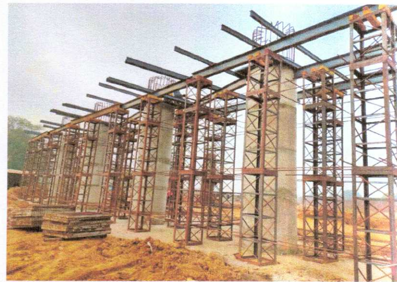
344+383 FLYOVER, PIER LIFT AND PIER CAP SHUTTERING AND STAGING WORK IN PROGRESS
