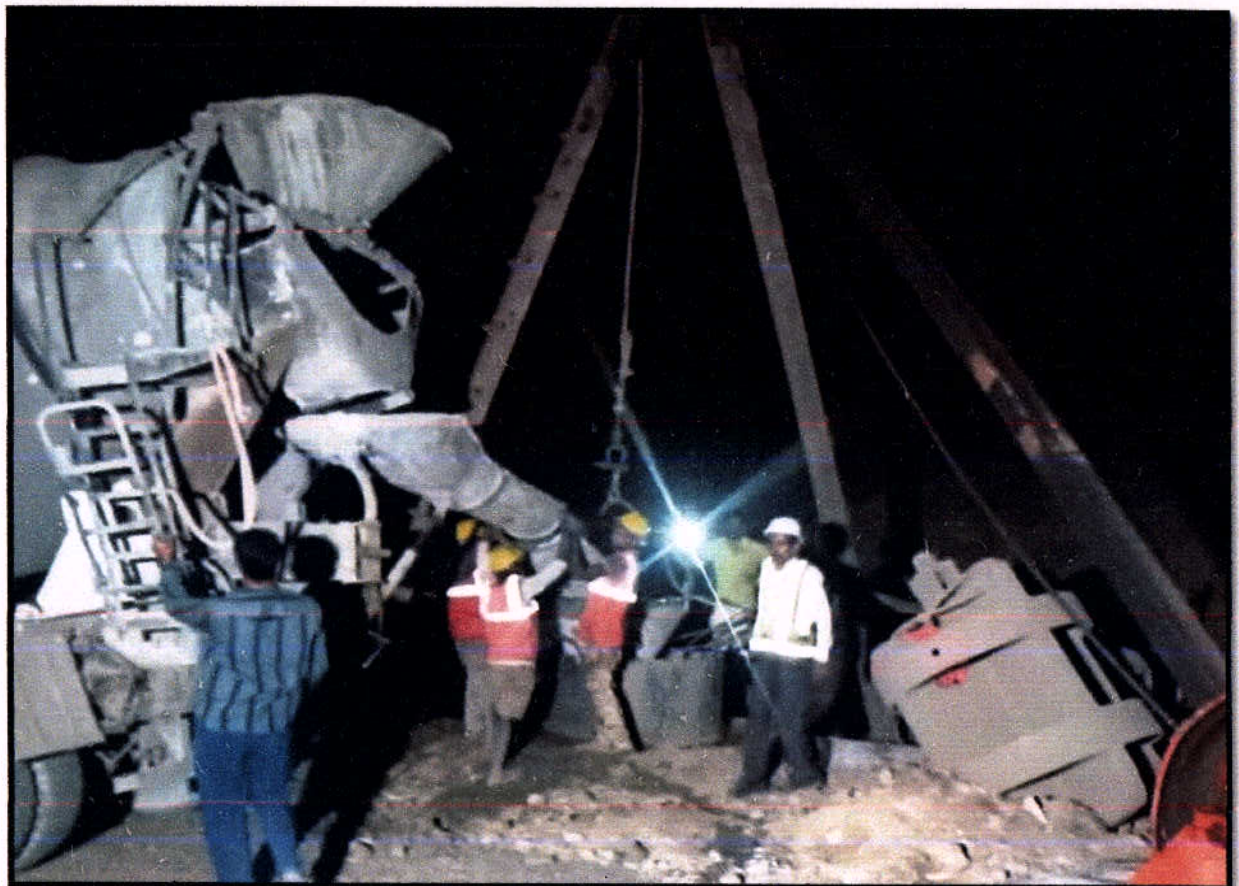
Concrete Pouring for Pile No-04 of Pier P-2 of MJB Ch 57+127 (RHS)
