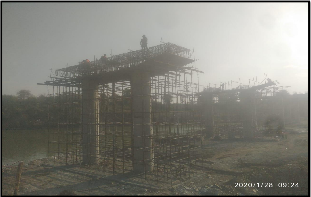
Pier P-4 to P-5 Pier Cap Reinforcement Work at MJB at Ch 36+070
