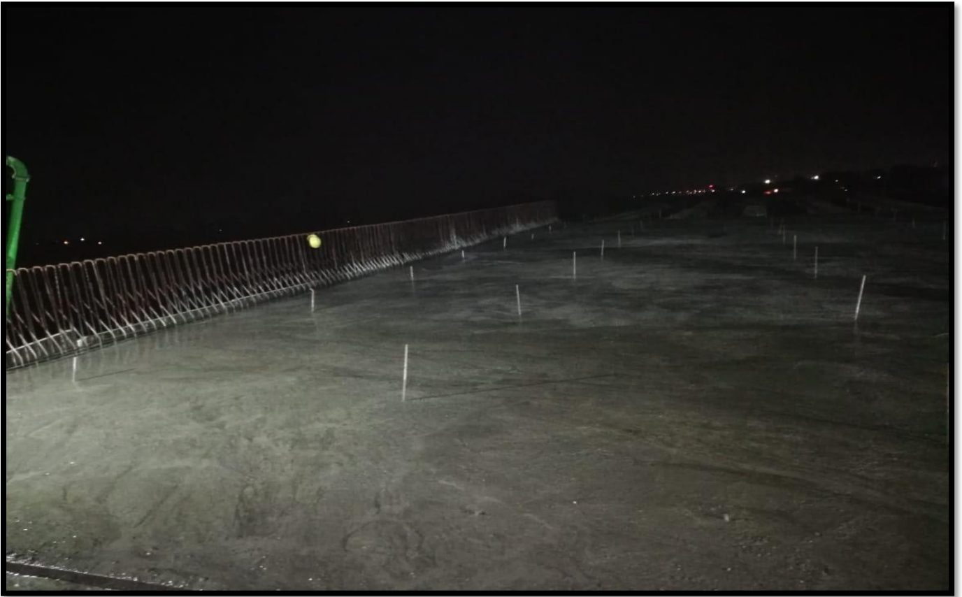
Deck Slab of Pier P-5 to Pier P-6 of Elevated Highway @ Km 47+830
